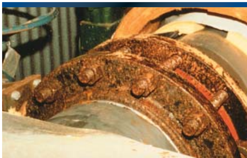
Corroded flange under absorbent insulation.
