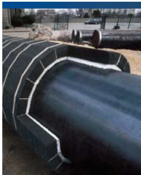
FOAMGLAS® insulation was installed as part of a composite insulation system. It incorporates a one-inch layer of fibrous glass felt material directly around the pipe, covered with FOAMGLAS® insulation.
