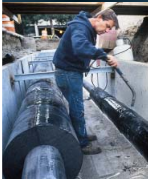
StrataFab® sections were installed in succession and butted against one another with PITTWRAP® butt stripes at the interfaces, and heat sealed.
