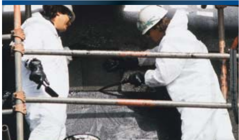
FOAMGLAS ® insulation—in 2" (50.8 mm)-thick, 12" x 18" (304.8 mm x 457.2 mm) blocks—being applied to a petroleum storage tank at a West Coast refinery. Industrial applications include pipelines as well as vessels of all types.
