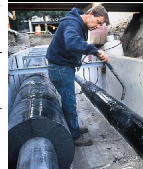
StrataFab® sections were installed in succession and butted against one another with PITTWRAP® butt stripes at the interfaces, and heat sealed.
