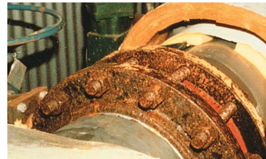
Corroded flange under absorbent insulation.
