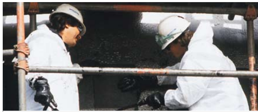
FOAMGLAS® insulation—in 2" (50.8mm)-thick, 12" x 18" (304.8mm x 457.2mm) blocks—being applied to a petroleum storage tank at a West Coast refinery. Industrial Applications include pipelines as well as vessels of all types.
