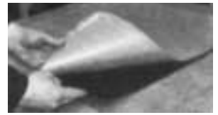
2 Starting at edge of PITTWRAP® jacketing lap seal, apply butt strip half way around, lapping two inches on each side of butt joint.
