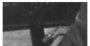
12 Heat remaining half of butt strip, pull it around, and make lap seal.
